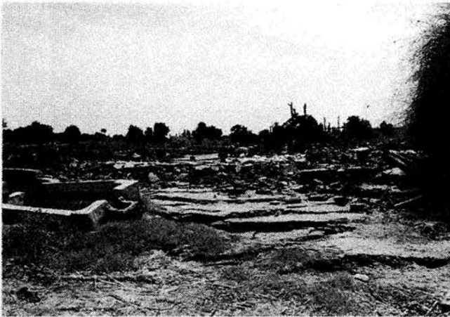
Photo 2.8. Right-stepping fractures causing total destruction of a farmer's house just on them. Looking southeast.
