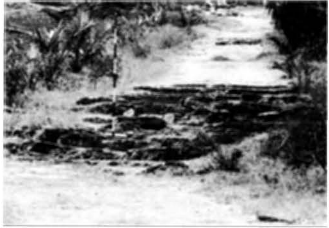
Photo 2.10. A close-up view of the north-facing steps in Photo 2.9. The fractured ground slumped about a meter to the north by densely spaced extensional faults.
