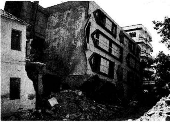
Photo 2.22. A view of collapsed reinforced concrete building tilted 90° during the present quake at Bhuj.
