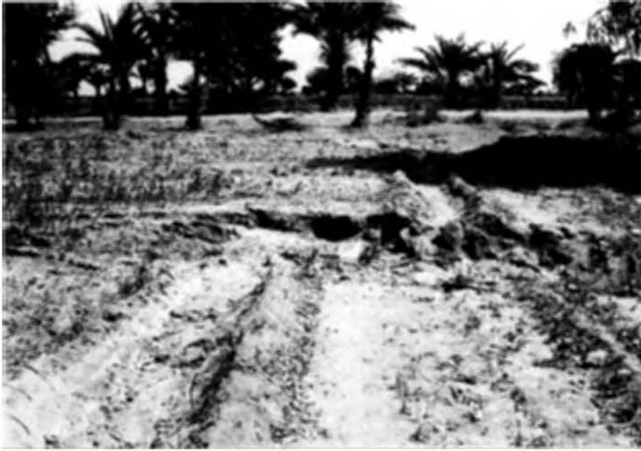
Photo 2.7. An apparent right-lateral offset of an irrigation channel along an N-S striking fracture in an agricultural field, looking east. The ground in front of the fracture is locally moved northward due to lateral spreading in a highly moist soil close to a pond in the upper slope to the south.
