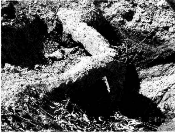
Photo 7.3. Foundation of collapsed five-story RC building.
