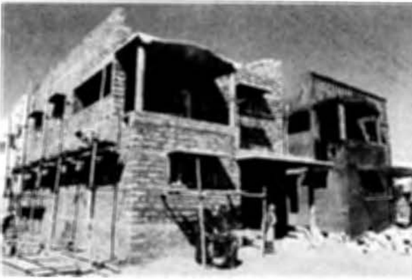
(a) Left side: Before finishing the outside wall, Right side: After finishing the wall
