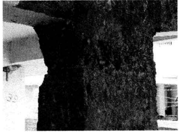
Photo 7.4. Honeycomb concrete can be seen above the construction joint.
