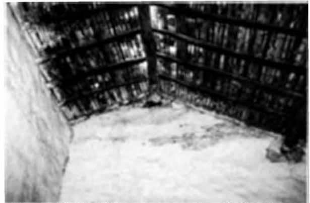
Photo 7.26 Roof damage caused by tile slipping
