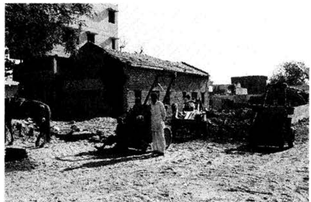
Photo 7.28 Separation of the adjacent walls of a single story masonry dwelling
