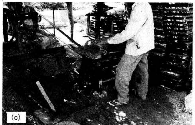
(c) Compression, compaction and vibration of the mortar for forming the blocks
