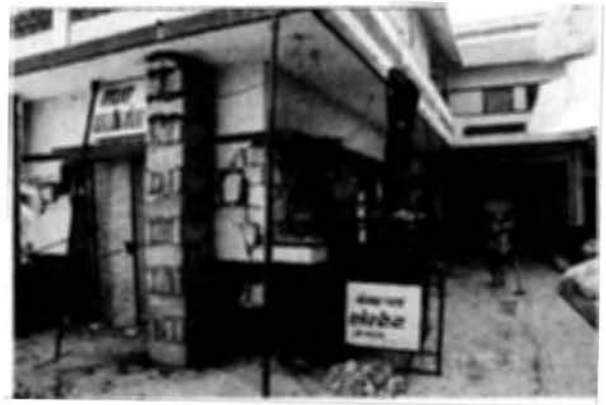
Photo 7.38 Microtemor measurements at a two-story brick masonry house damage level G4
