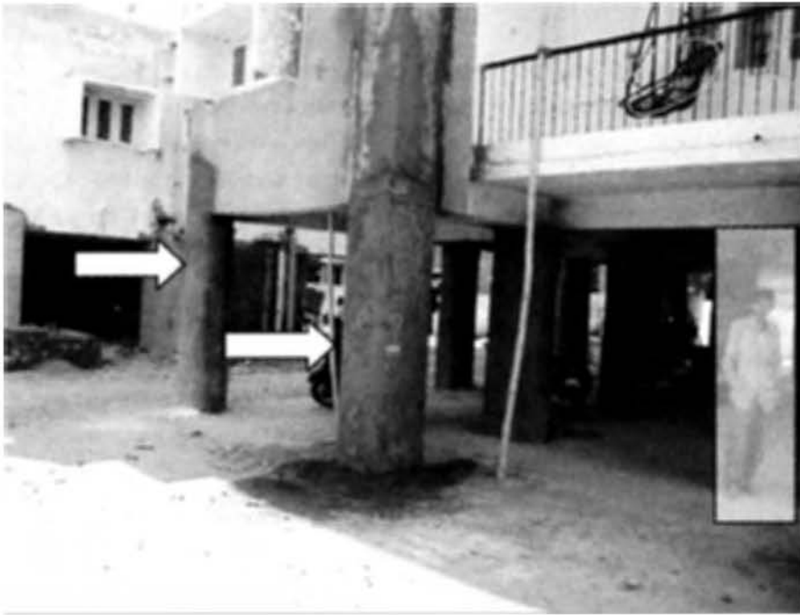
Photo 7.41 Repair work was done by shotcreting mortar on the damaged columns of the first-story.
