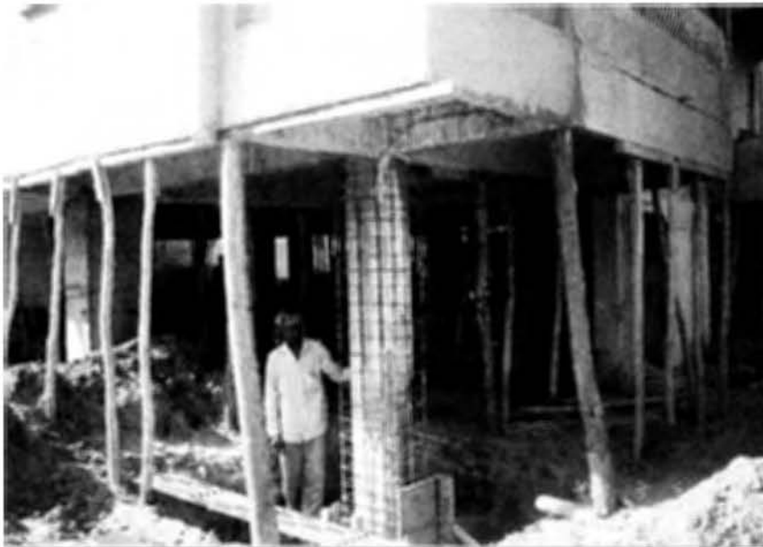
Photo 7.42 Repair work under progress of the damaged columns of the open-first-story of a 4-story apartment building in Ahemadabad. Old concrete from the columns had been chipped-off with additional reinforcement before concrete jacketing.
