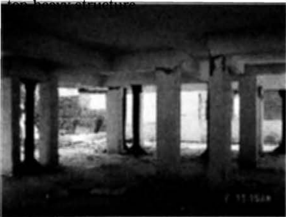
Photo 7.6. Columns are arranged in an irregular manner and the aspect ratio is large.
