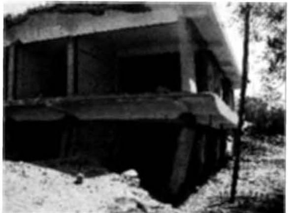
Photo 7.7. RC building in Bhachau collapsed in a side sway mechanism.
