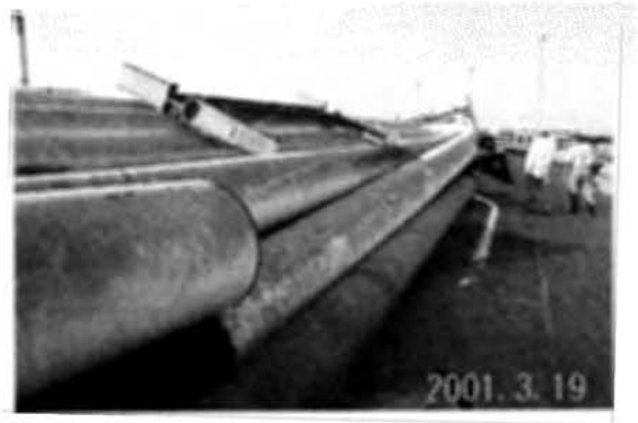
(c) damaged pipelines with collapsed steel frame
