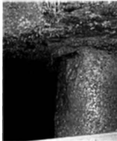
(a) chipped pile head
