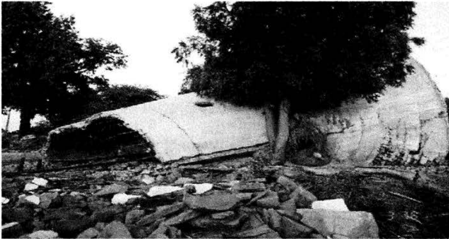
Photo 8.16. Collapsed water tank in Chobari village
