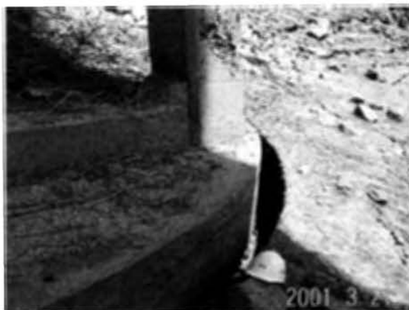
Photo 8.6. Gap between foundation and surrounding soil at Rudramata bridge
