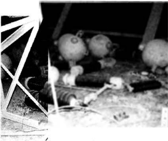
(b) damaged circuit breaker
