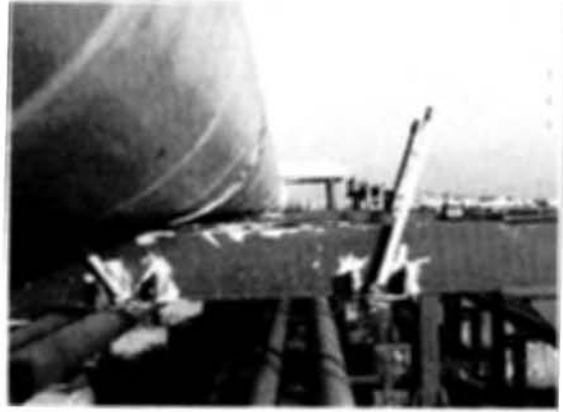
(a) broken fixtures
