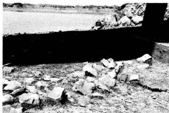
(b) crack due to lateral spreading
