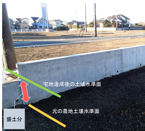
Figure 14 The difference of surface levels before and after land formation for new housing construction (photo taken by Author)
