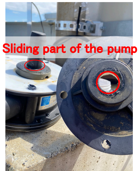
Fig. 3.23 Photo shows sliding part of the pump using in the air pumping system pictured on March 20, 2020.
