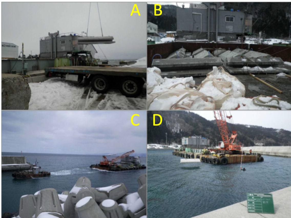
Fig. 4.13 Installation of the concrete blocks for sea cucumber aquaculture. A, loading concrete blocks onto the barge on March 5, 2018; B, ten concrete blocks loaded on the barge on March 7, 2018; C towing the barge from Aomori Port on March 7, 2018; D installation of concrete blocks onto the mouth of fishing port. on March 13, 2018.
